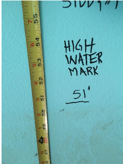
Figure 2 - Use a permanent marker to note the water height in each room. Photograph the mark along with a tape measure showing the height.
