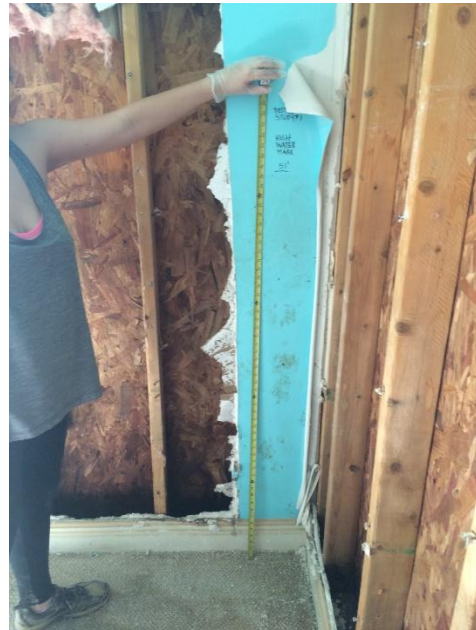
Figure 3 - Leave one vertical section that includes the wall material and base board as well as special conditions (built-in shelves) . Step back and take a photo showing the wall and tape measure. Use high resolution photographs.
